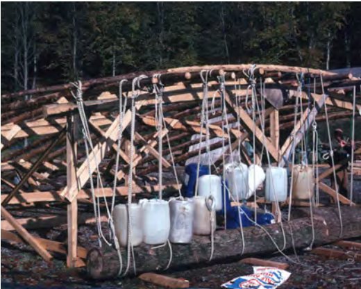
Above: A lattice of roundwood thinnings forming the Westminster Lodge is bent into shape.
