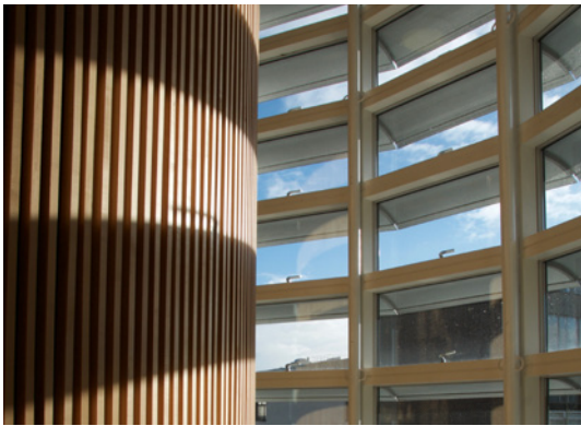
Above: Bespoke louvres shed water from the facade whilst providing shade from solar gain and glare.
